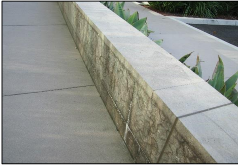
Photo # 57 Hollow installation, efflorescence from joint resulting from moisture trying to escape
