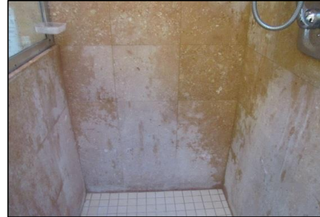
Photo # 52 Badly etched stone shower - correct: grinding, refinishing and seal
