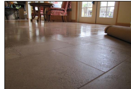
Photo # 56 Another view of too many coats of topical sealer on a textured granite floor
