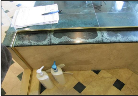
Photo # 49 Lack of slope, moisture evaporation causing spalling - correct: remove and replace using TCNA guidelines
