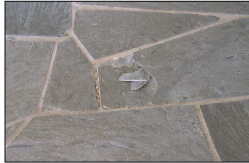
Photo # 50 Pressure on edges causing cleavage in stone to break off - partially hollow tile at the edge - correct: wet or dry sand the slate until smoother and fill void in with adhesive, then rearout
