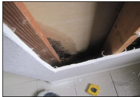
Photo # 58 Shower pan holding water and wicked off the walls past the membrane
