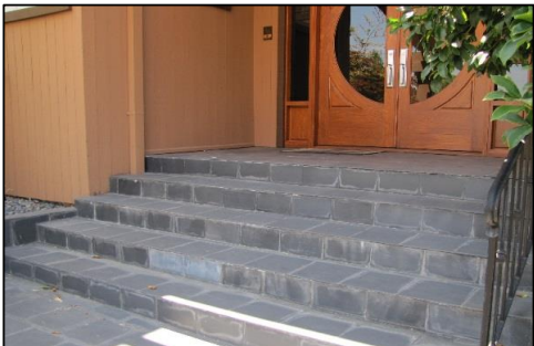
Photo # 103 Efflorescence in slate
