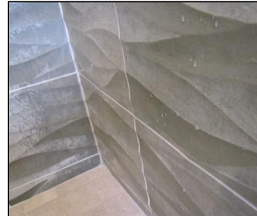
Photo # 64 Improper specification of material - very porous material in a wet area - correct: multiple sealing applications on multiple days
