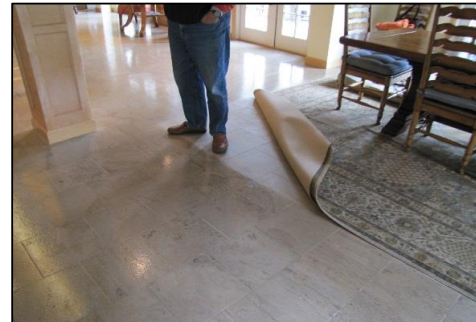
Photo # 54 Multiple coats of topical sealer on a textured granite floor - correct: carefully strip the floor, allow to thoroughly dry and use an impregnator
