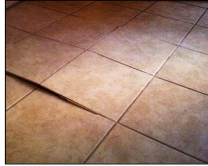
Photo # 98 Tenting - remove and replace affected tiles. Add movement and/or expansion joints per industry
