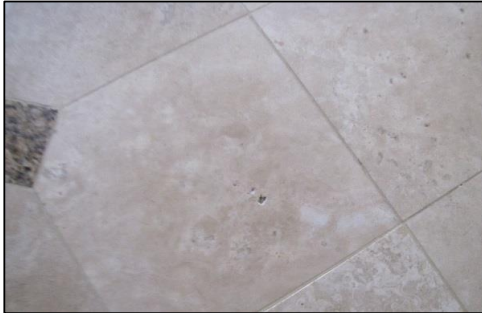
Photo # 59 Holes in travertine - correct: clean, prep and fill with epoxy
